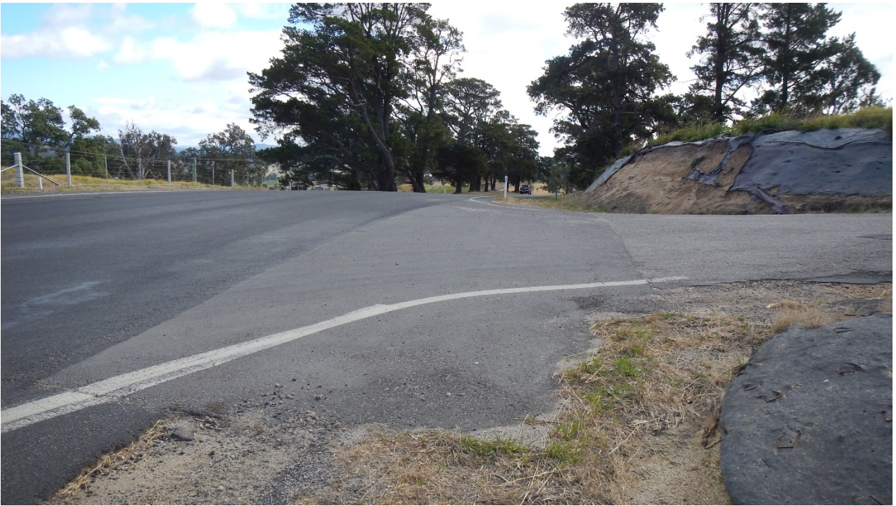
Figure 3 Corkhill intersection with Newton Road demonstrating in excess of 200 metres sight distance to the north
